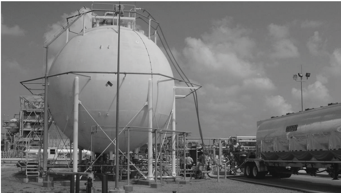
FIGURE 2. The 218,000 L liquid hydrogen tank is shown with its annulus being filled with glass bubble insulation from an over-the-road pressure differential trailer. The flexible fill and vent hoses can be seen draped over the right side of the tank.
